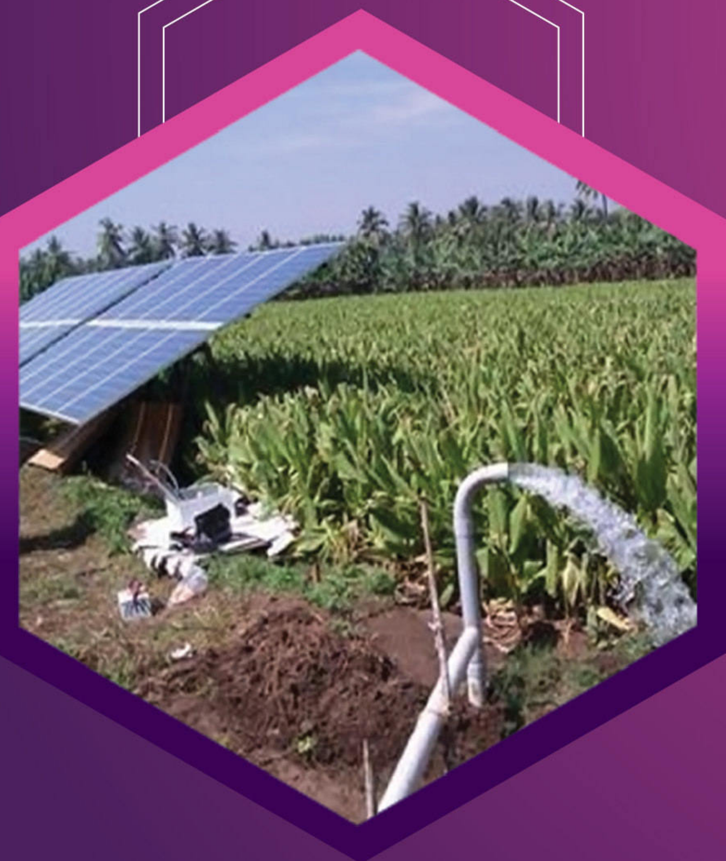
Solar Irrigation Pump System
